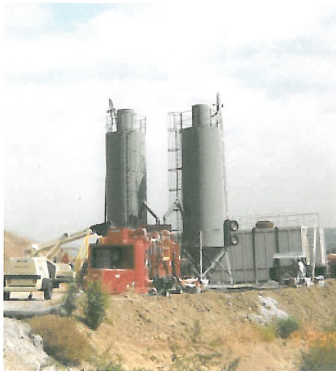
Figure 2. Central Grout Mix Plant
