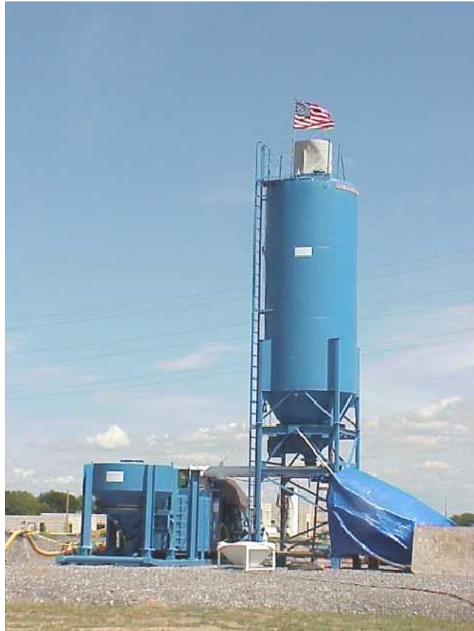
Figure 5. Grout mixing plant
