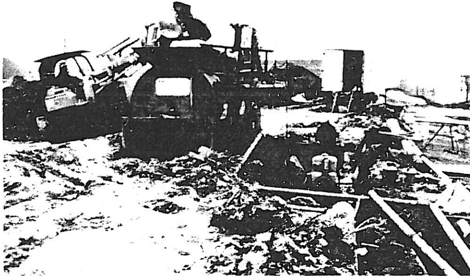
5. Akron Project - Batch Plant
