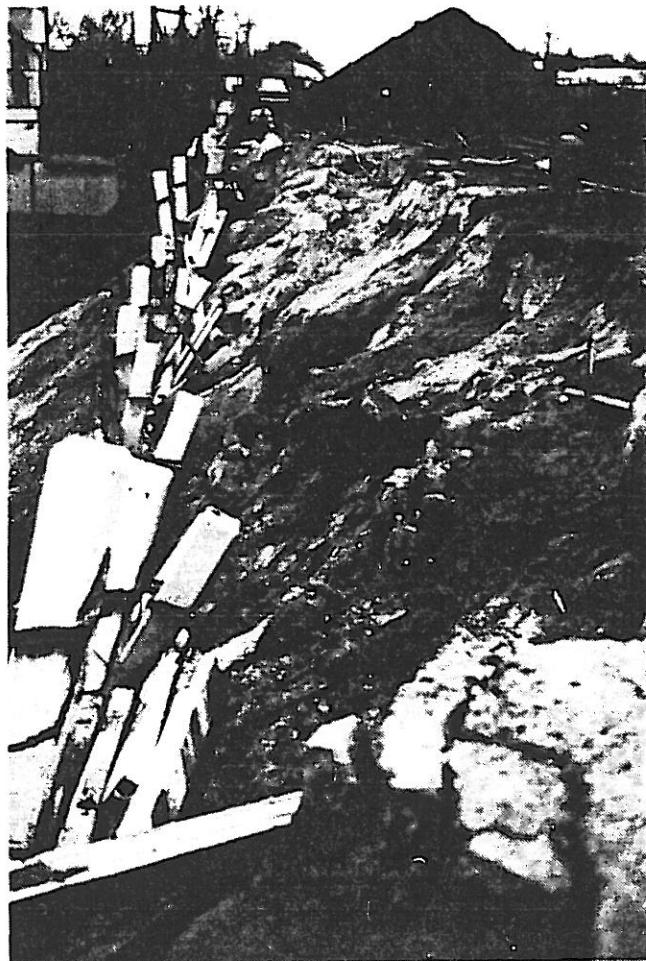
2. Akron Project -- Slope Failure Caused by Burning
