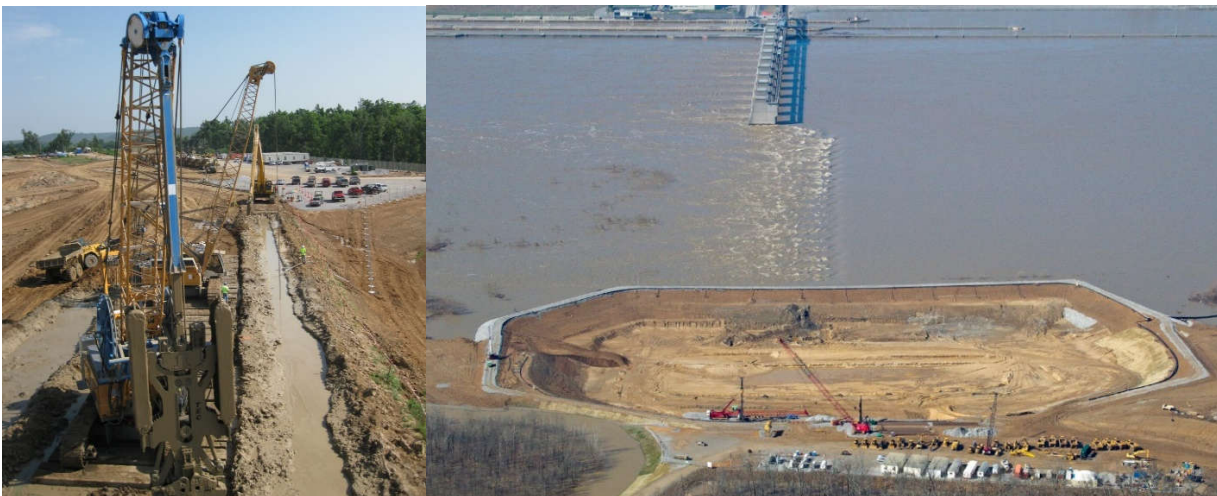
Figure 4. World’s deepest circumferential slurry wall, constructed to a depth of 56 m (185 ft) deep. On left: with backhoe (background) and clamshells (foreground), on right showing final embankment adjacent to a flooded Ohio River for a 100 ft deep hydroelectric plant excavation (photos courtesy of Geo-Solutions Inc.)
