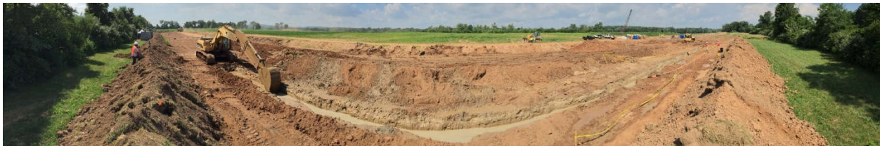
Figure 1. Photograph of slurry trench excavation from NSF Research Site at Bucknell University (photo courtesy of Geo-Solutions, Inc.)
