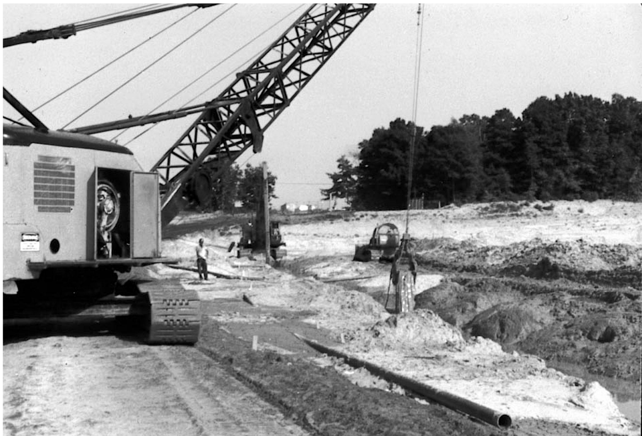
Figure 3. Photo of SB slurry wall construction showing long stick excavator, clamshell and bulldozer backfill mixing
